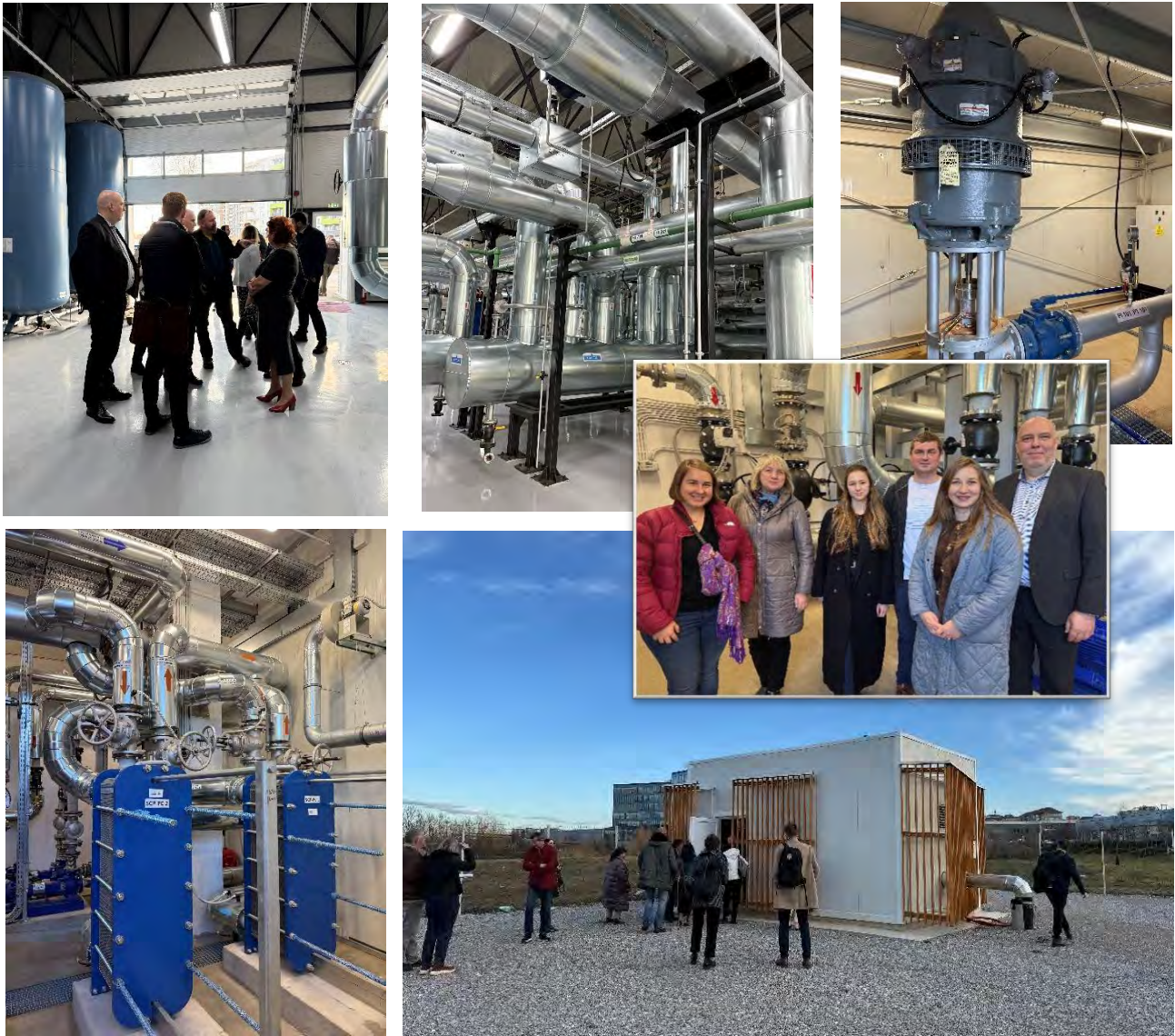
Visited facilities of the general heating system in Oradea
