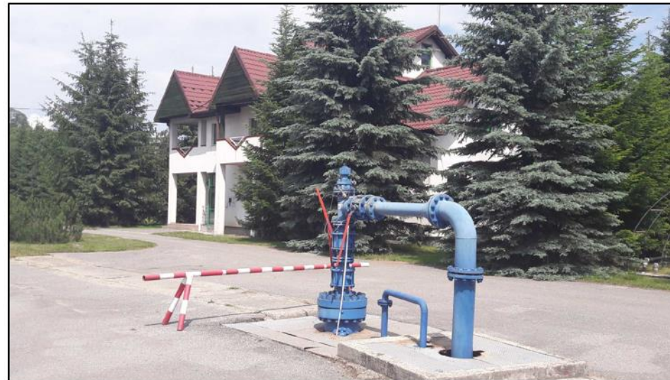
Podhale Region: MEERI PAS Geothermal Laboratory 1st in Poland Experimental Geothermal Plant (since 1993)
